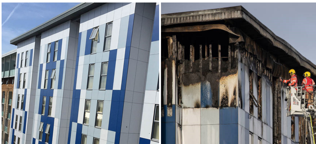
Figure 27. The HPL cladding of the Cube before [72] and after the fire in 2019 [73]
